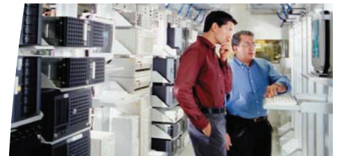
Can be integrated into high density racks.
