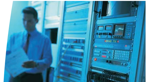
Servers, data storage and network equipment.
