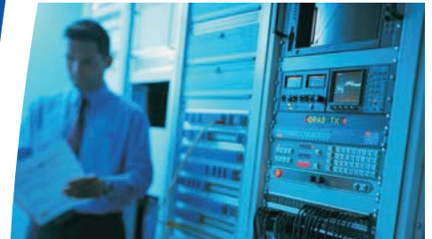
Servers, data storage and network equipment.
