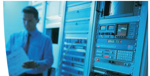
Can be built in to high density racks.
